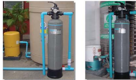
Installations of W250 filters with pressure pumps and water reserved tanks
